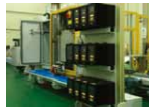
Electric Control Rack
